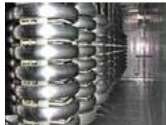
Inside a valve enclosure with IGBT valves Photo courtesy of ABB
